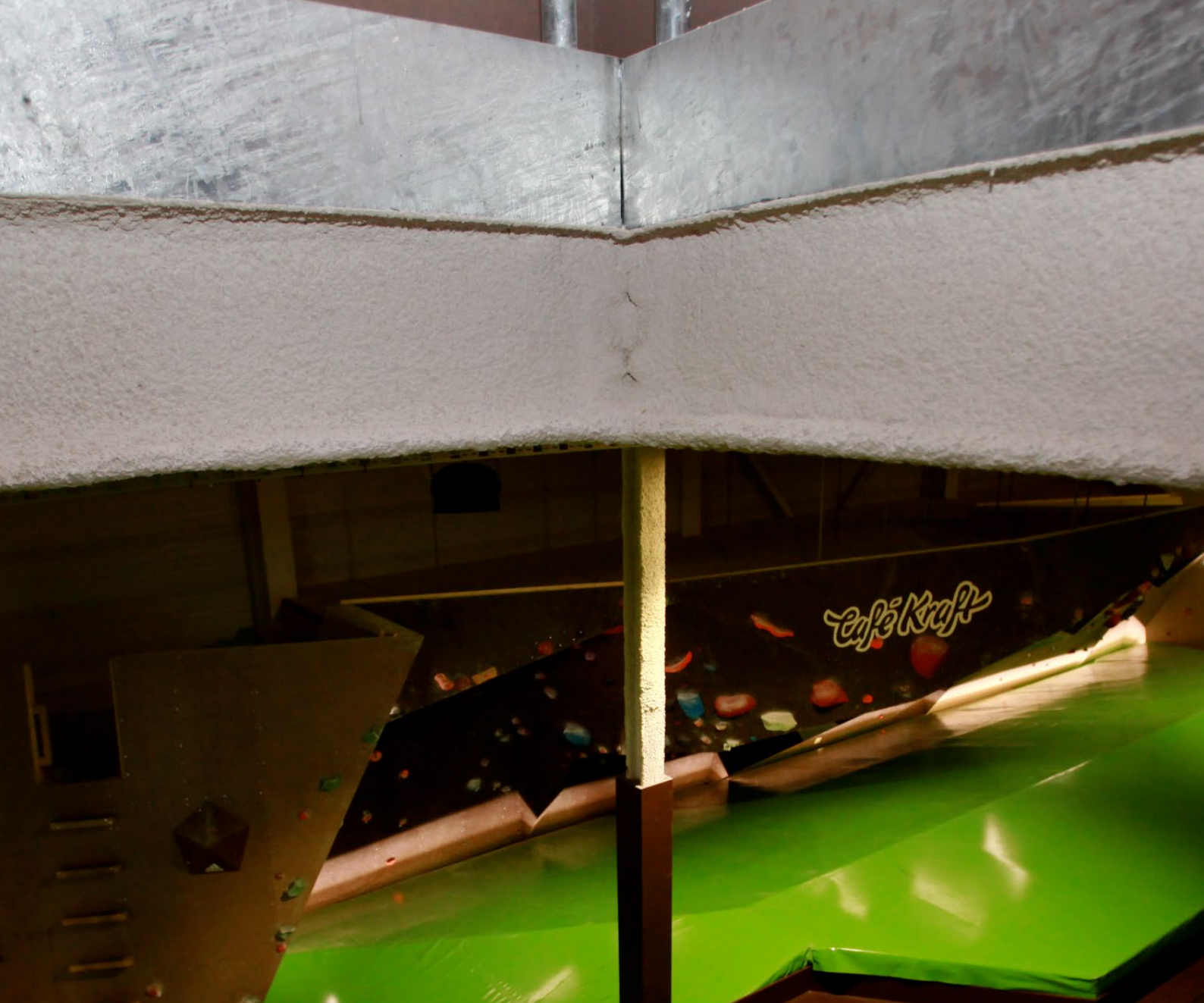
MP 75 Fire Fire Protection Gypsum Plaster
